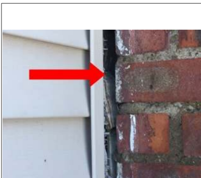
Flashing has pulled away from the chimney - recommend repair
