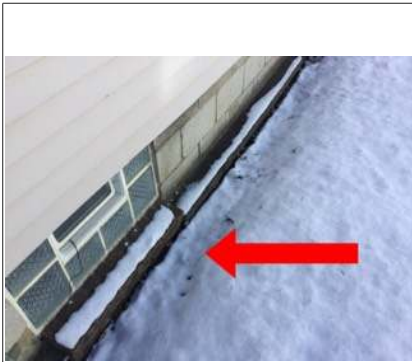
Low areas of grading next to the foundation recommend adding additional soil and slope away from foundation
