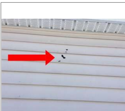
Small cracks in siding needs repaired/replaced
