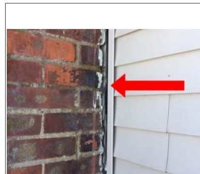
Flashing has pulled away from the chimney - recommend repair
