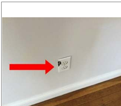
Receptacle cover needs replaced
