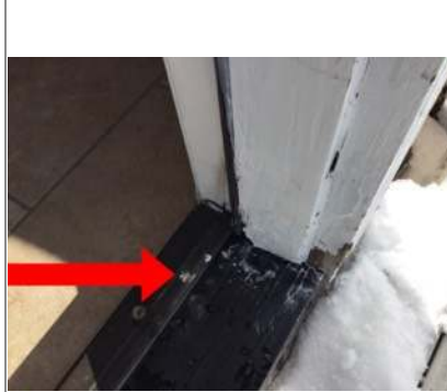
Back door threshold needs repaired by a licensed contractor.
