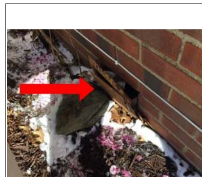
Clean out rusted and needs replaced by a licensed contractor.
