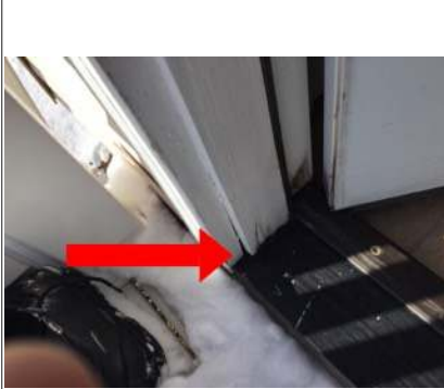
Front door needs painted to prevent wood rot.
