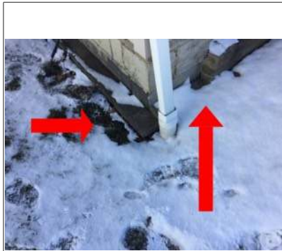
Low areas of grading next to the foundation recommend adding additional soil and slope away from foundation
