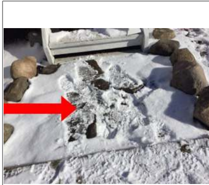
Safety hazard ground is not level, needs to have a contractor repair/replace
