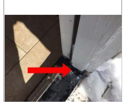
Back needs painted to prevent wood rot.
