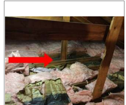
Needs more insulation installed in attic
