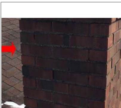
Loose bricks or stones create a safety hazard recommend repair by a qualified chimney specialist
