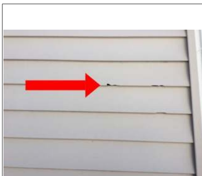
Small cracks in siding needs repaired/replaced
