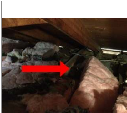
Need more insulation installed in attic
