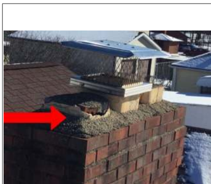
Chimney crown is loose - recommend licensed contractor repair
