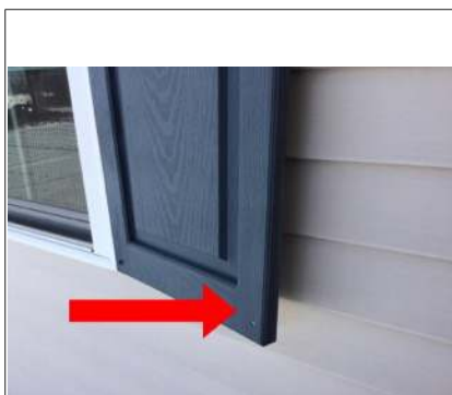
Loose needs fixed
